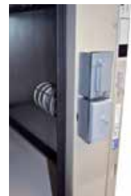
Lights and receptacles
